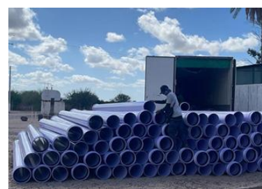
Purple pipes for water reuse
