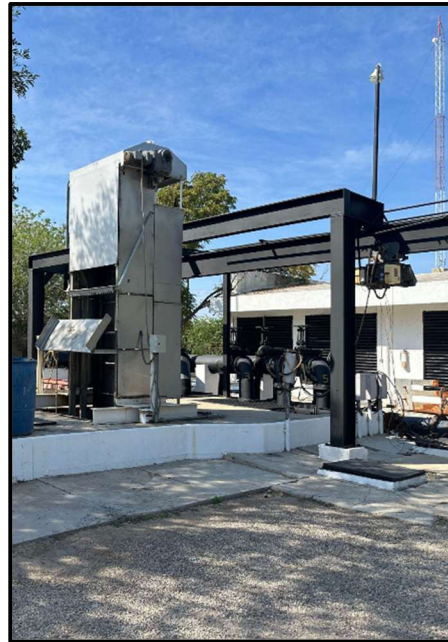
Figure 2-3. Las Alamedas Lift Station
