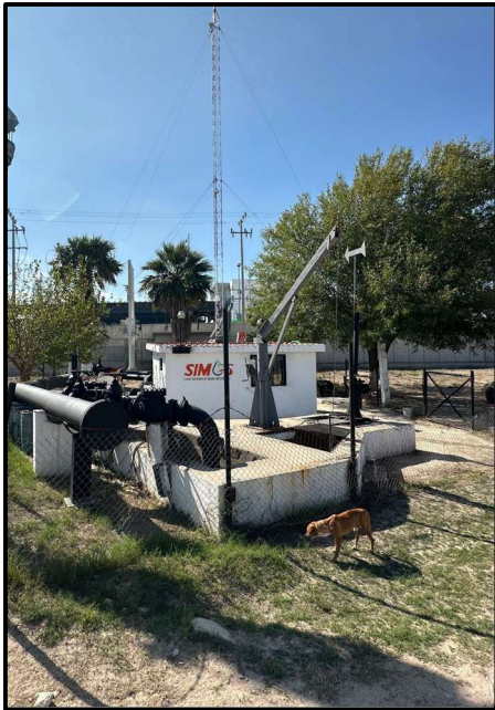
Figure 2-2. Puente Internacional Lift Station
