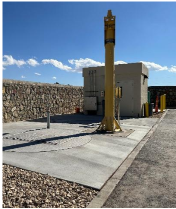
Lourdes Estate wastewater system
